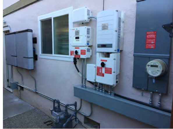
2 Storage Batteries, Inverter with EV Charger, Storage Inverter, Solar-Ready Service Panel
