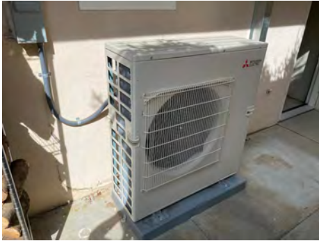
Heat Pump HVAC
